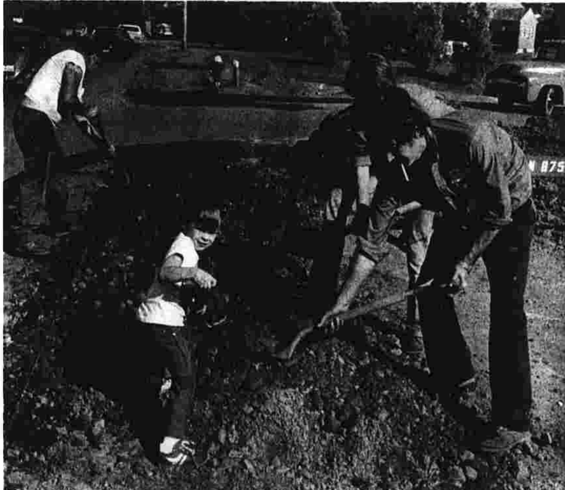
Sidewalk job a family affair Putting in sidewalks is a family affair at the corner of Rt. 83 and Regan Rd. in Vernon. Three-year-old Greg Hurlburt lends a hand to (left to right) his grandfather, Norman Chapman of Norman Chapman and Sons Construction Co.; his uncle, Clifford Hurlburt, and his father, Michael Hurlburt. (Herald photo by Dunn)
